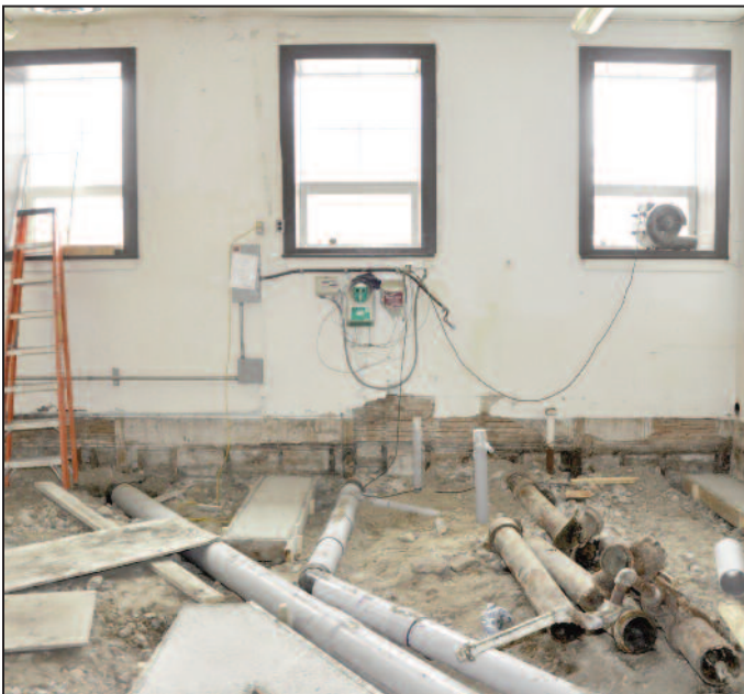
KITCHEN RENOVATIONS – The abbey kitchen floor was removed and replaced by a new floor during April of 2017.
