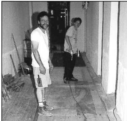
Br. Randy Senecal renovating the basement of the college with Devin Schlosser.
